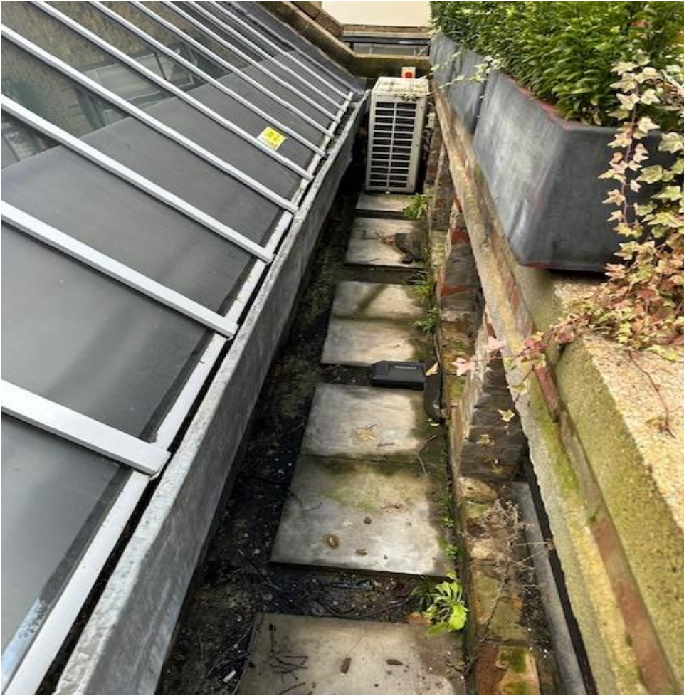
Figure 3. Showing the semi-covered enclosed, it's proposed to cover this area with top panel/weatherhood
