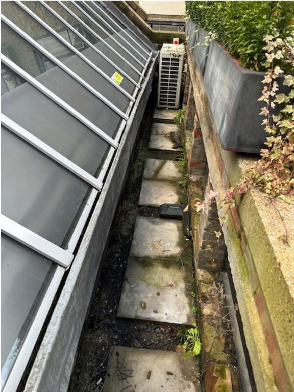
Image 4. Showing a close up of the Plant enclosure.
