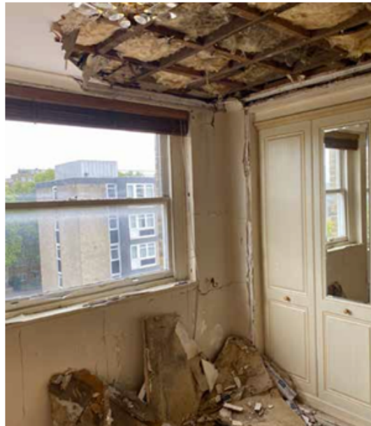
Collapsed ceiling at third floor bedroom
