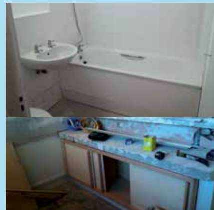
New bathrooms and kitchens being fitted at a flat in Alexandra and Ainsworth Estate
