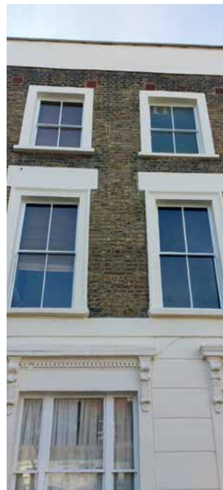
Completed external painting and window repairs at one of our homes on Bassett Street
