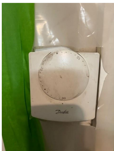
Typical mechanical thermostat installed within a property
