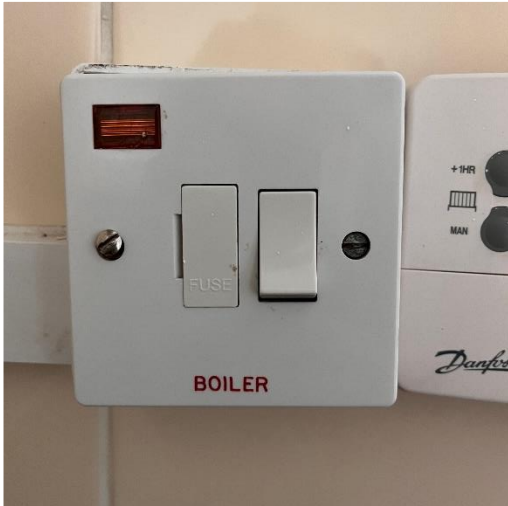
Boiler supply wall switch turned off
