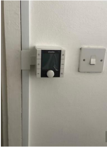
Trench heater thermostat turned off
