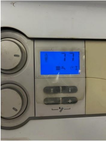
Boiler display screen on
