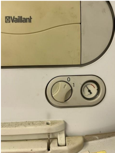
Boiler supply internal switch turned off
