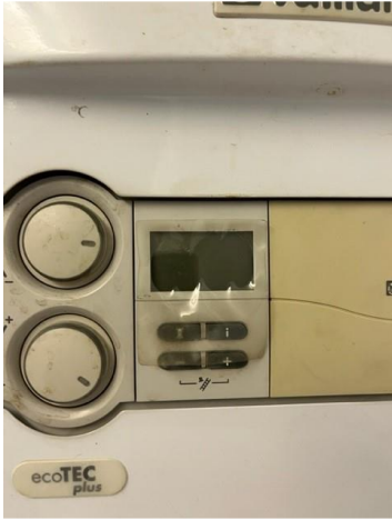
Boiler display screen off
