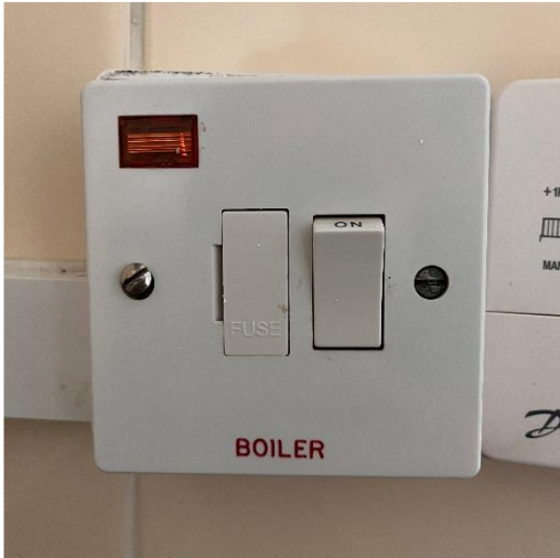
Boiler supply wall switch turned on and the neon light is illuminated to indicate this
