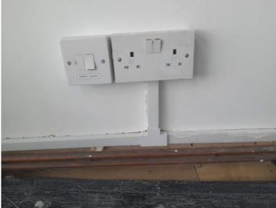
Trench heater wall switch in the off position
