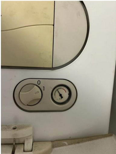
Boiler supply internal switch turned on
