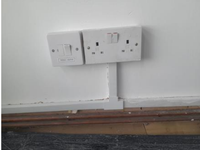
Trench heater wall switch in the on position
